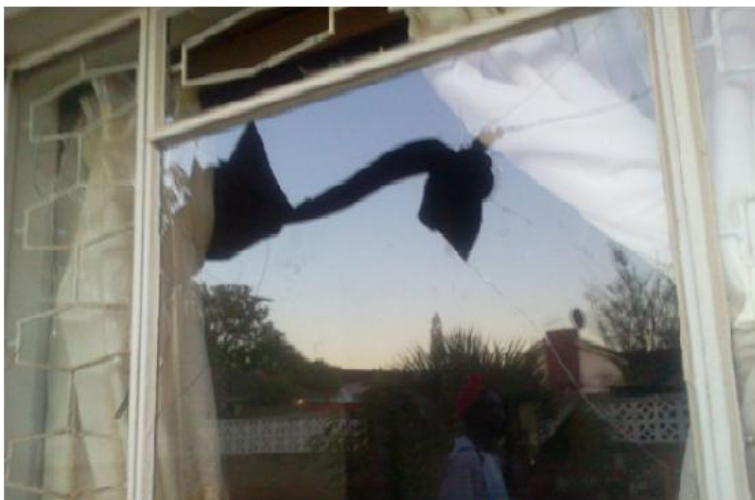
Broken window at Dorcas Sibanda's house
