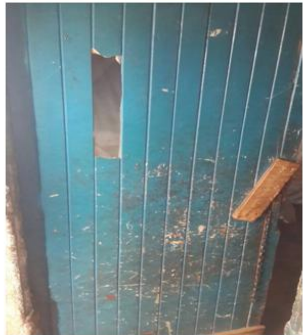
Front and back doors vandalized at John's premises
