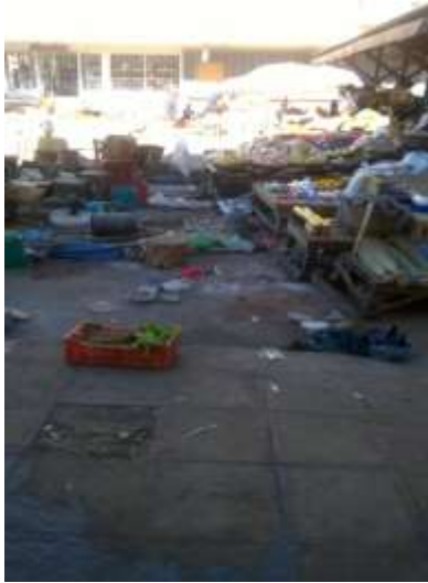
Informal traders' stalls demolished in preparation for the rally in Mutare (Picture by ZPP)
