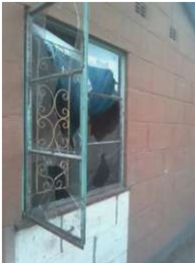
One of the windows damaged by suspected Zanu PF supporters (Picture by ZPP)
